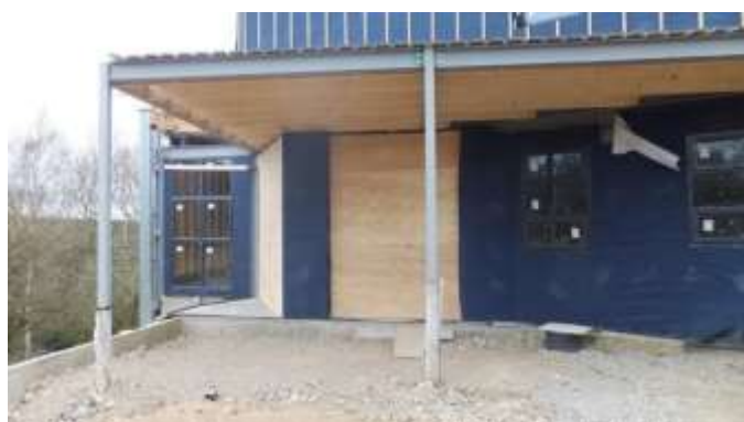
The outdoor eating area is now really taking shape even if the entrance is now boarded up for security.
