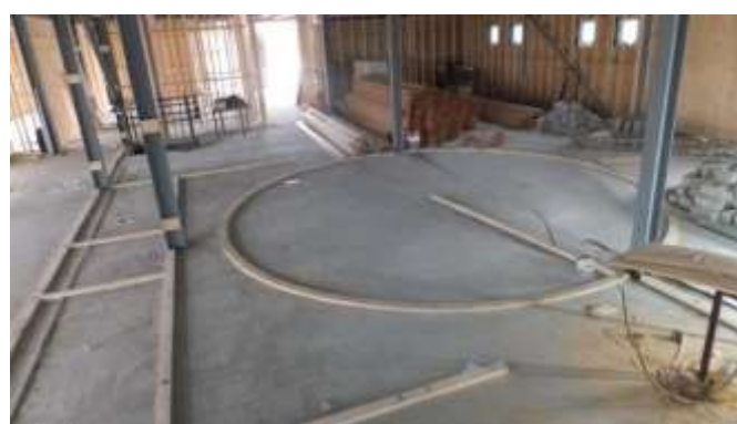
The circular foyer and adjacent stores have now been set out. Studwork shown in the distance is for the store and county office.
