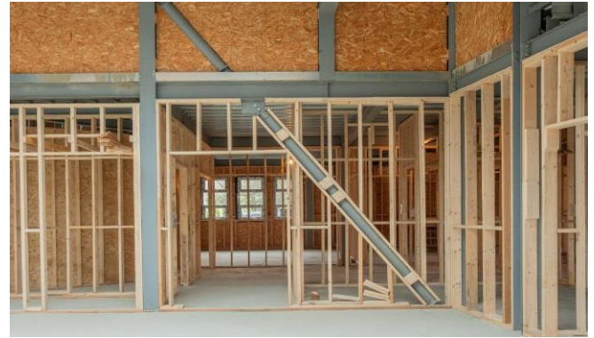
Walls are starting to be fully insulated and the basement floor has also been completed.
